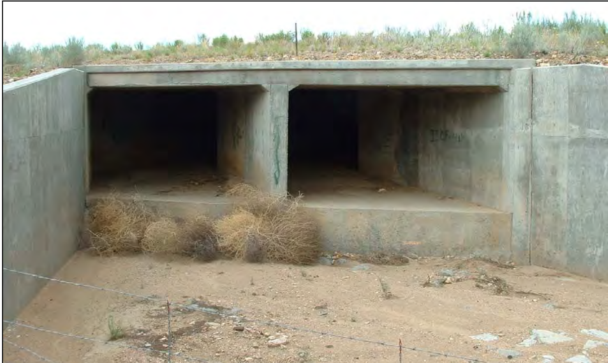
Figure 14: Looking south-southeast from waypoint 096, two 8x12 ft culverts under I-40 are unusable to most species due to a 3 ft pour-off (top) and an angled exit (bottom).
