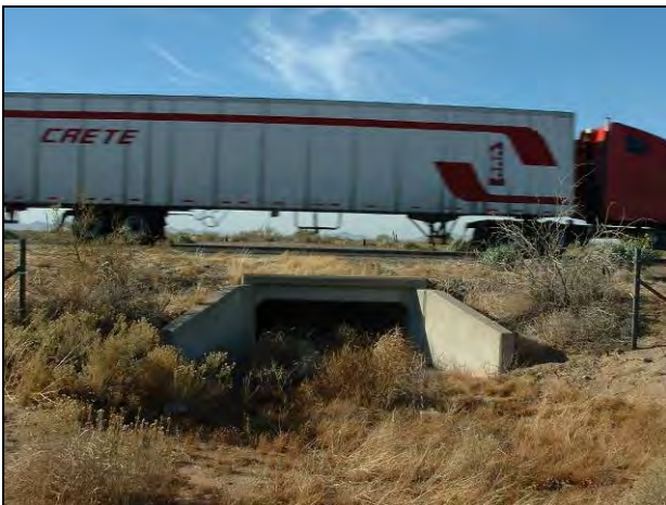
Figure 15: A small 4 x 6 ft cement culvert filled with tumbleweeds (azimuth: 228) occurs at waypoint 92.
