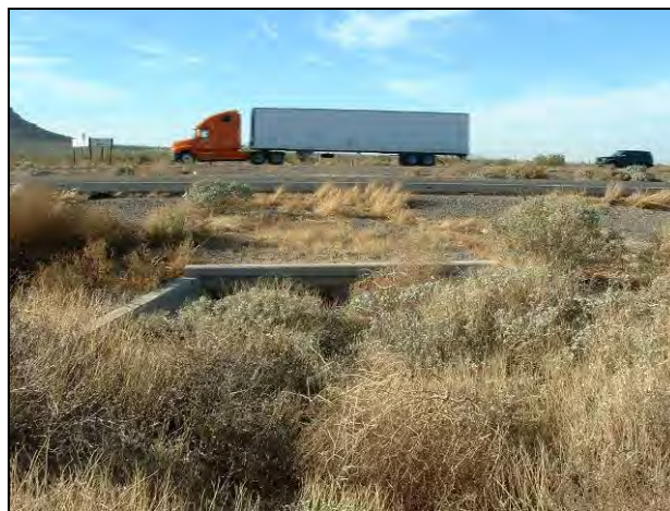
Figure 13: The entrance of this small box culvert north of Picacho Peak State Park has been blocked with vegetation (waypoint 90, azimuth 24).
