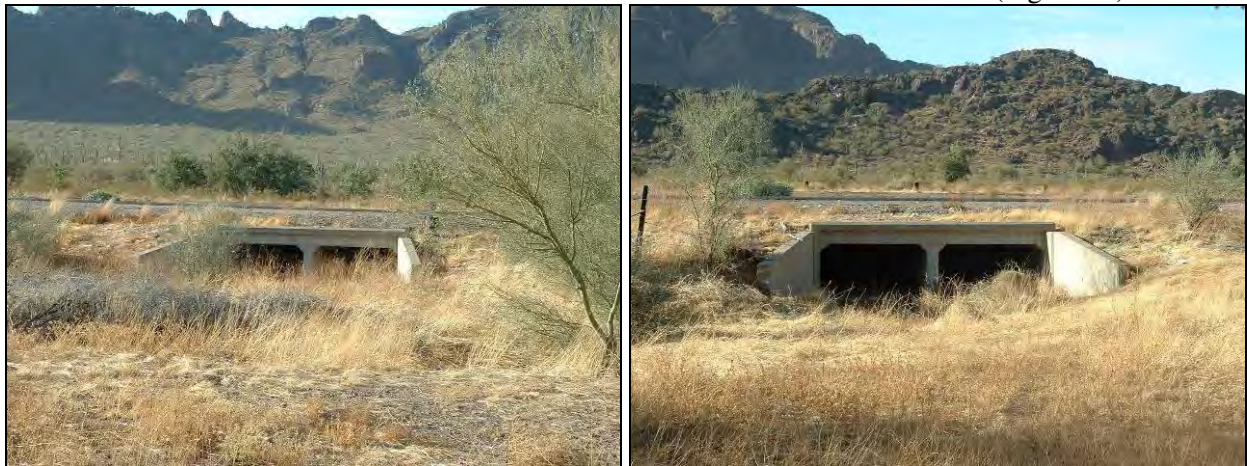
Figure 12: Two examples of twin-span 4 x 6 ft culverts found in the Ironwood – Picacho strand of the linkage design (Left: waypoint 88, Right: waypoint 89. Azimuth on both photos: 220).
