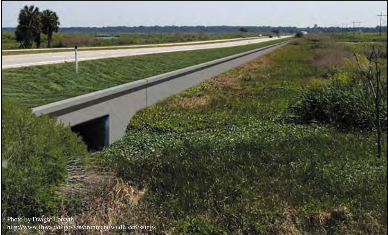
Figure 11: The protruding lip on a concrete wall will stop snakes and other reptiles and amphibians from scaling the wall, and the concrete is less permeable than wire fencing. The Paynes Prairie Ecopassage (Florida) successfully directs animals to the undercrossing (culvert) and has reduced road mortality by over 95%.
